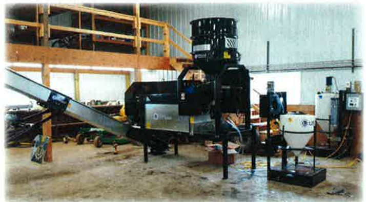
Quality Grain Services recently installed a USC LPX 2000 seed treatment machine.
